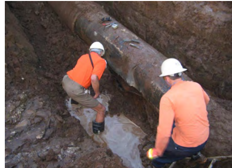
The Labrador Lane 24-inch main ruptured in 2008 400 feet away from the Interstate. This pipe crosses under the Interstate and is not in a casing.
