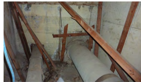
16-inch concrete cylinder potable water pipeline inside bridge girder under I-8 at Victoria Drive.
