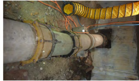
10-inch Asbestos Cement Potable Water pipeline located inside bridge box under I-8 at Tavern Road.
