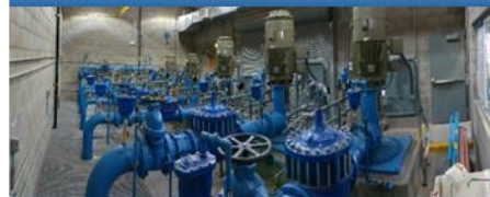
Navajo Pump Station
