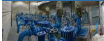
Navajo Pump Station
